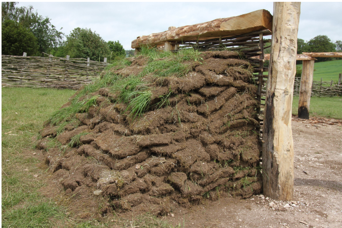
Fig. 3: Photograph of an embanked turf wall section during construction (photograph by the author).
